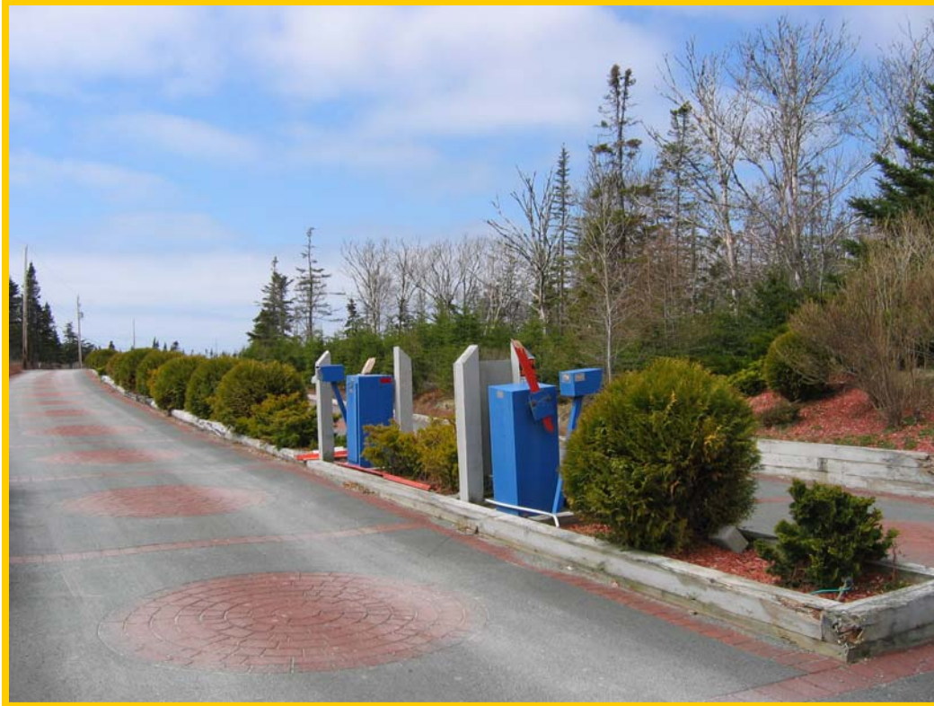
Figure 4. The lift arm gates at Abbecombec Ocean Village have been broken off and not replaced. [Source: J. Grant]
